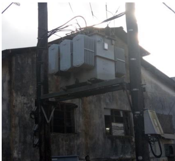
FIGURE 8: POORLY MAINTAINED TRANSFORMER, GADCO
