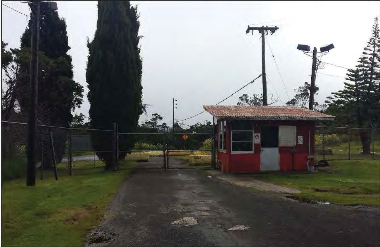
Perimeter Light _Q: Two green bulbs, with full shielding, located immediately southwest of the guard shack.
