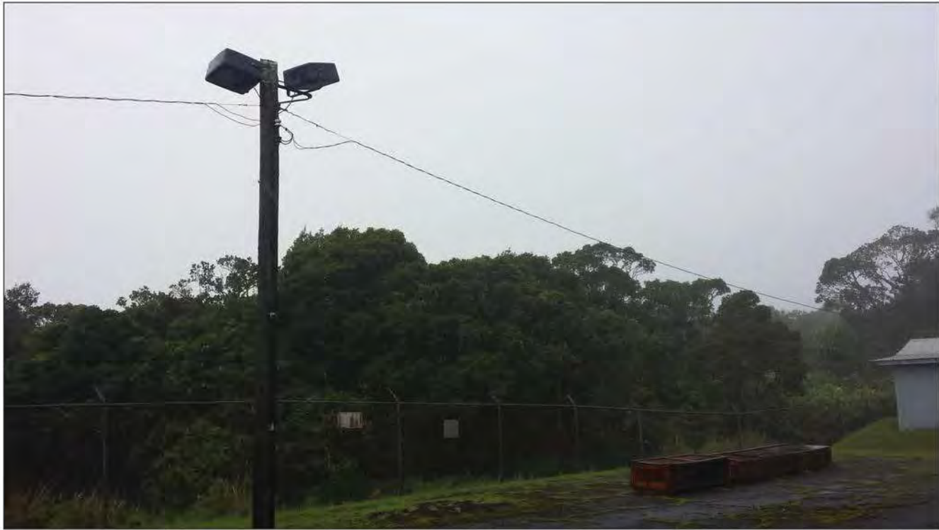
Perimeter Light _N: Two green bulbs, with full shielding, along the south fenceline.
