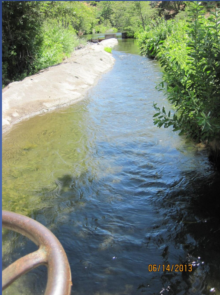
DCID ditch from stream to headgate
