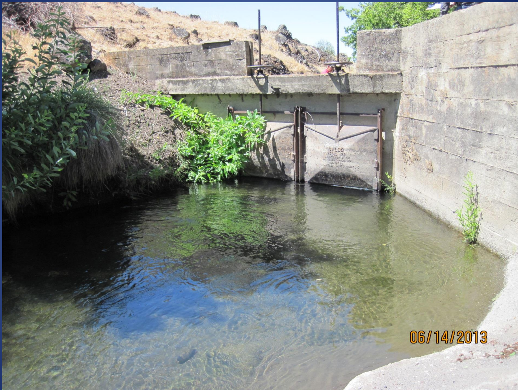
DCID headgate, upstream side
