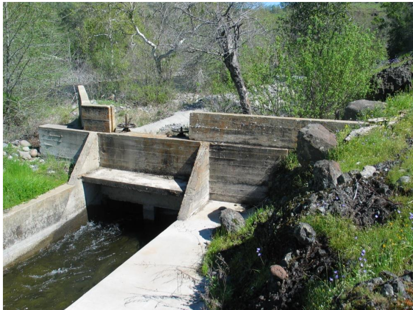
Figure 4. Headwall with two 48-inch vertical slide gates (March 11, 2005). Photo: DWR
