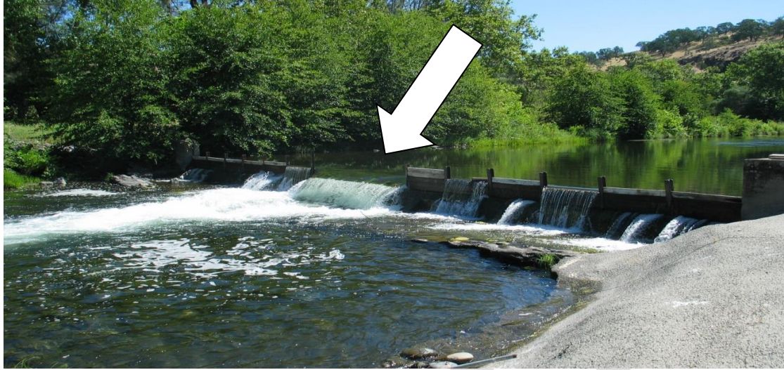
Figure 2. DCID dam without flashboards in the center section for fish passage (July 8, 2005, Deer Creek Flow = 135 cfs, DCID diverting 24 cfs).
