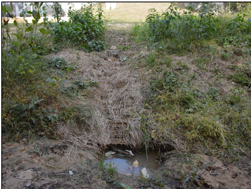
Photo 4. Headcut forming under soil matting. Hydrology likely coming from adjacent manhole and associated pipes.
