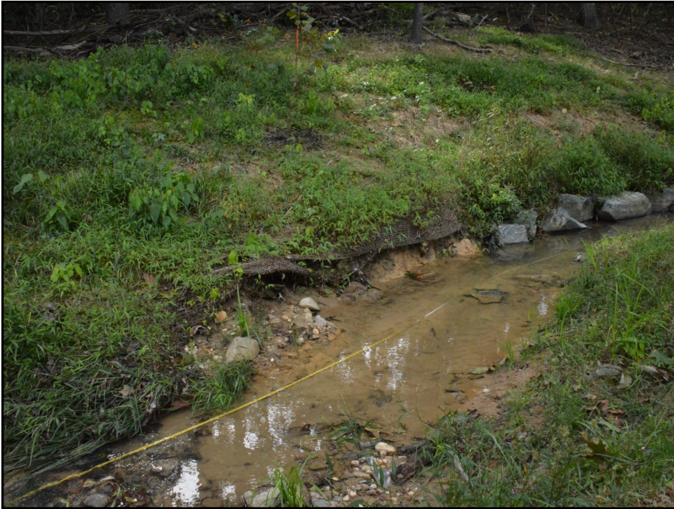
Photo 3. Ten to twelve feet of bank erosion at end of stone toe located along right bank (facing downstream) below culvert.
