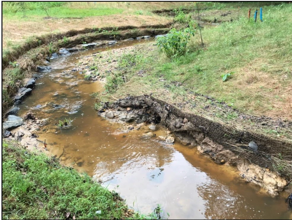
Photo 10. Post-storm inspection following 5.41-inch storm (facing downstream). Slight bank scour at end of stone toe.
