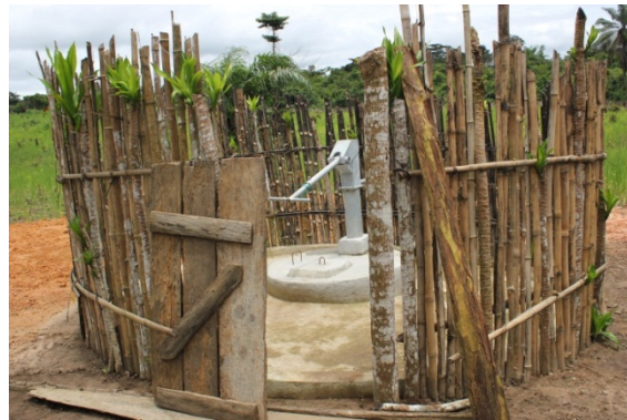
Hand-pump in Banamah, Bong County
